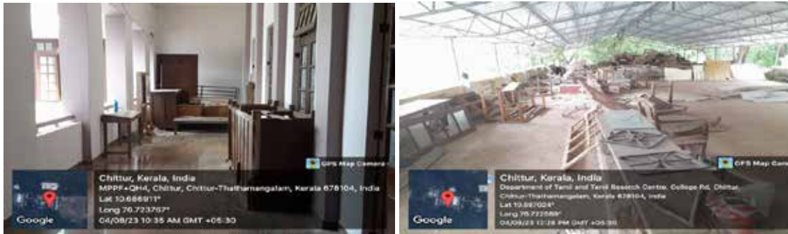
Broken furniture dumps in the room and roof of the college
