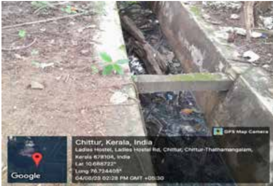
Open drain with liquid wastes, close to the ladies' hostel
